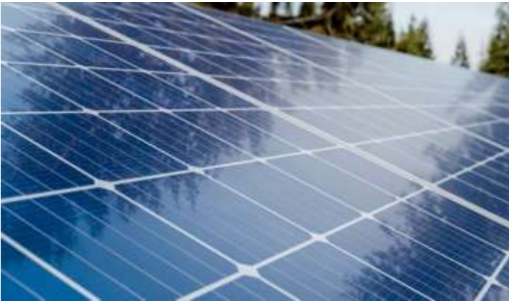
PV Inverter Monitoring
